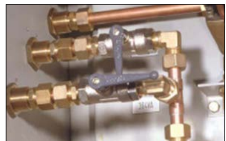
Modular assembly with copper tubing in a confined environment
